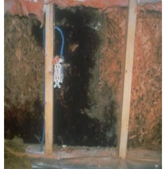
This is air leakage
