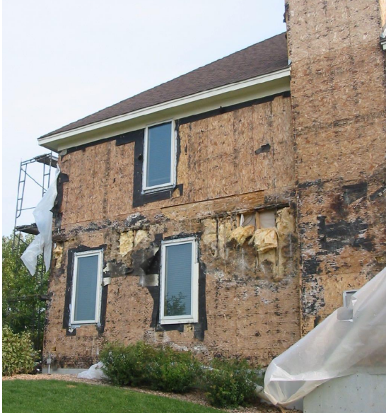
This is air leakage
