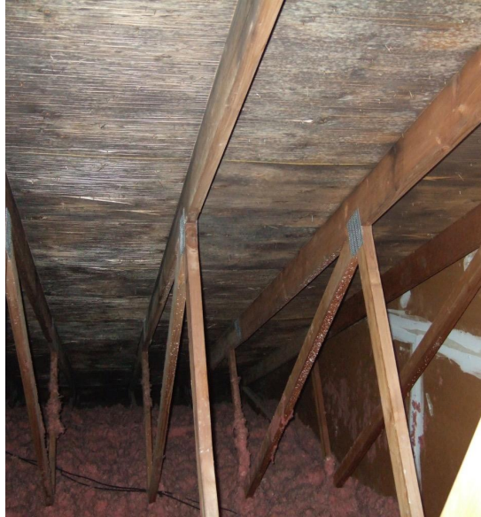
This is air leakage
