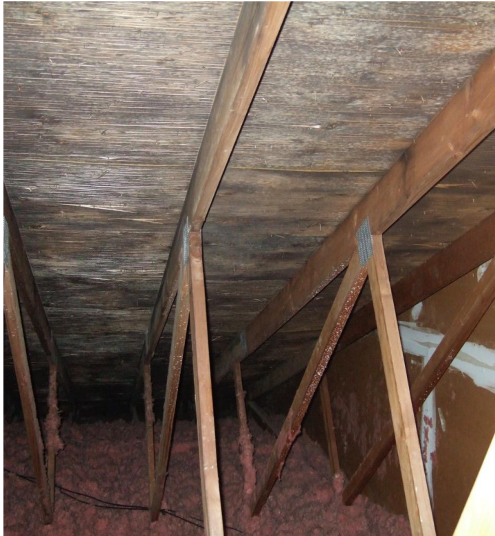
This is air leakage
