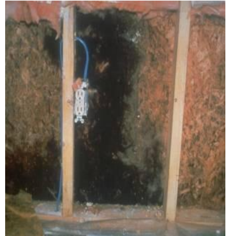
This is air leakage
