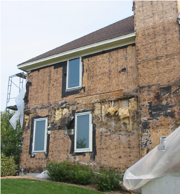
This is air leakage
