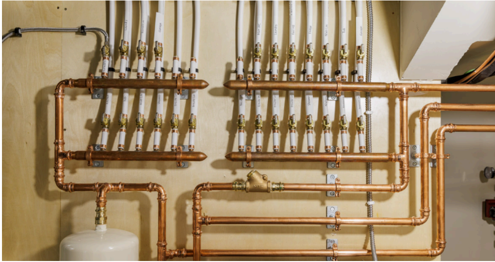
Figure 10 - The overall layout reflects a clean, organized installation of the manifold system
