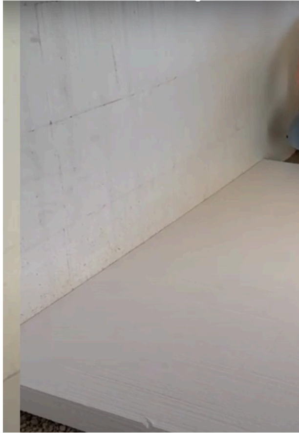
Figure 7 - ICF foundation wall and the continuous subfloor insulation in the basement.
