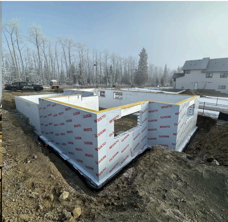
Figure 4 - ICF foundation wall panels with exterior membrane. Watch the video of the foundation wall pour here .
