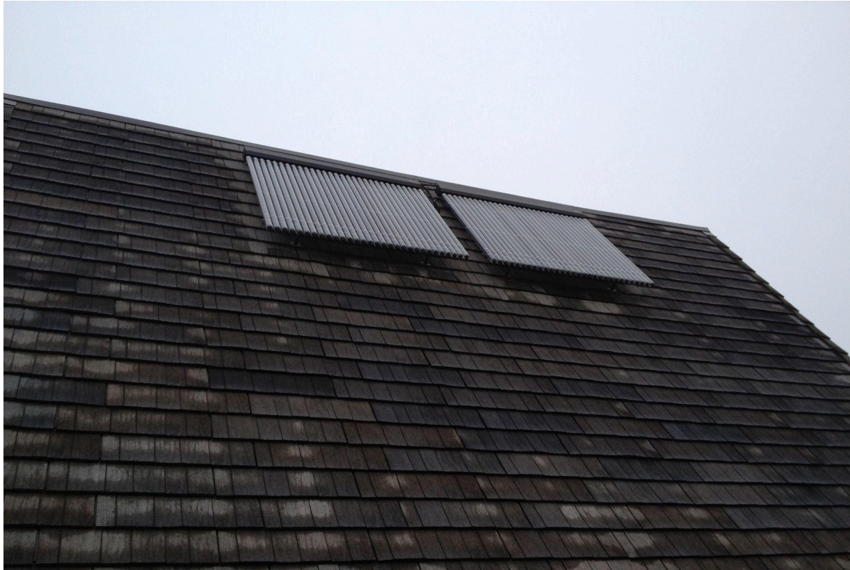
Solar thermal hot water heating system installed on a shingled roof, harnessing solar to provide efficient hot water heating year-round.
