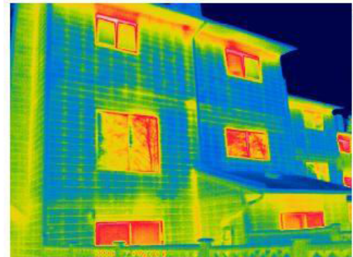
Infrared image of thermal bridging at studs, assembly interfaces, inside and outside building corners
